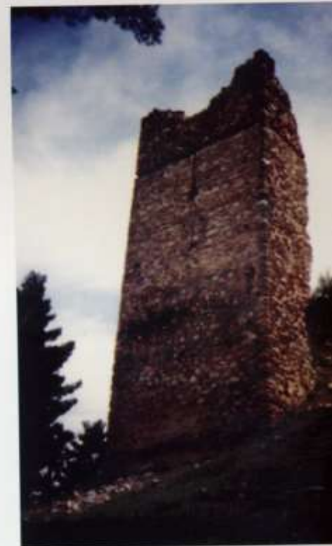
figure 22: Acropolis. West tower damaged by the earthquake in 1995.
