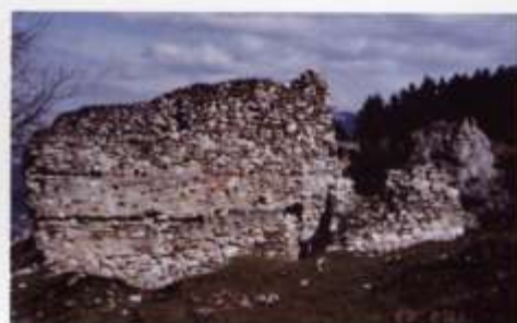
figure 14: Acropolis. Northwest part of the wall. Internal façade. Loose masonry at the upper part and rotten tie beams.
