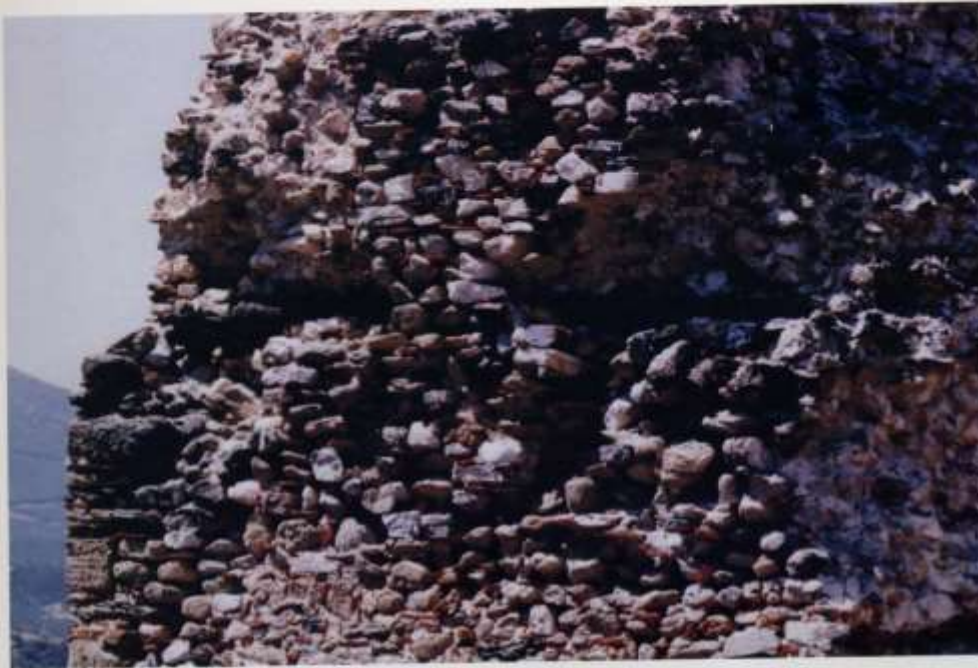
figure 21: Acropolis. Massive tower. Decayed joints and timber ties, behind the face of the wall.
