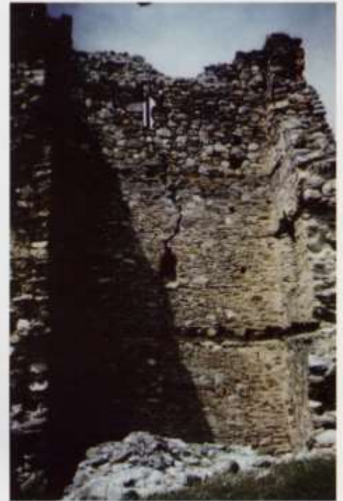
figure 24: West tower in 1995. The rate of decay is obvious.
