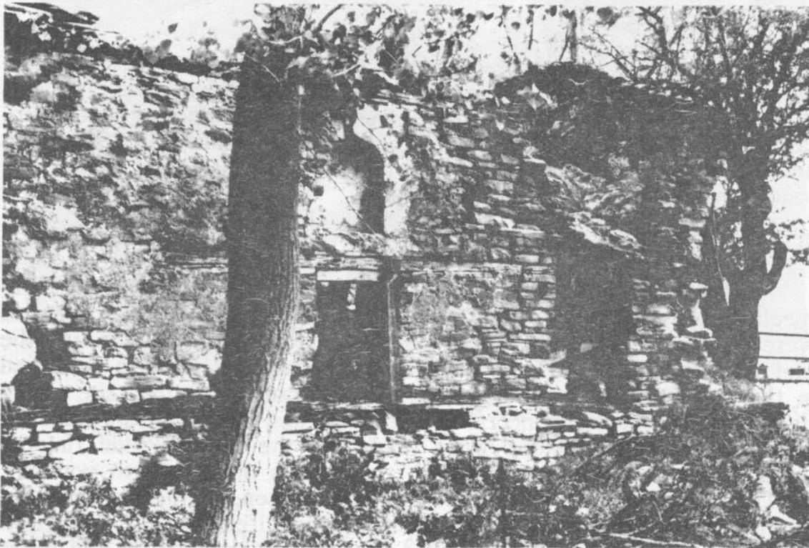
fig. 5 The south wall in 1981. The rebuild part of the east end can be distinguished, as well as the trees very close to the monument.
