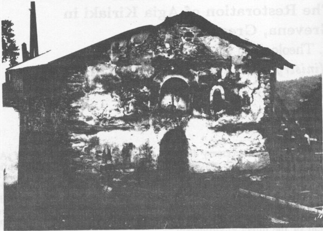
fig. 1 The church of Ag. Kiriaki in 1989 before the restoration works. Western facade.
